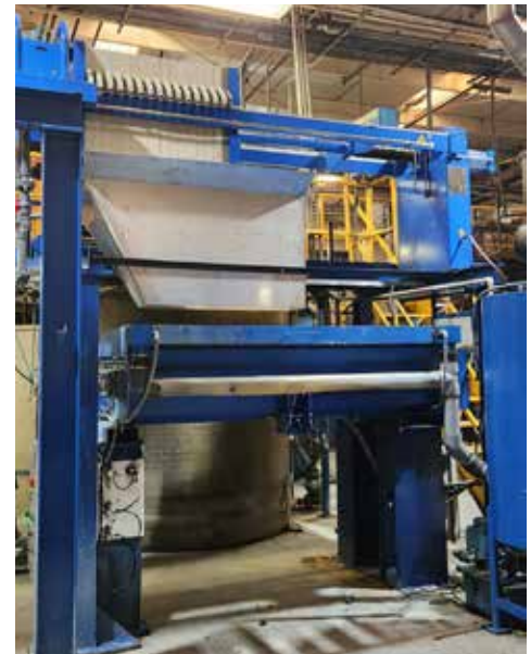
CONREC Sludge Dryer installed directly under CONREC Filter Press
